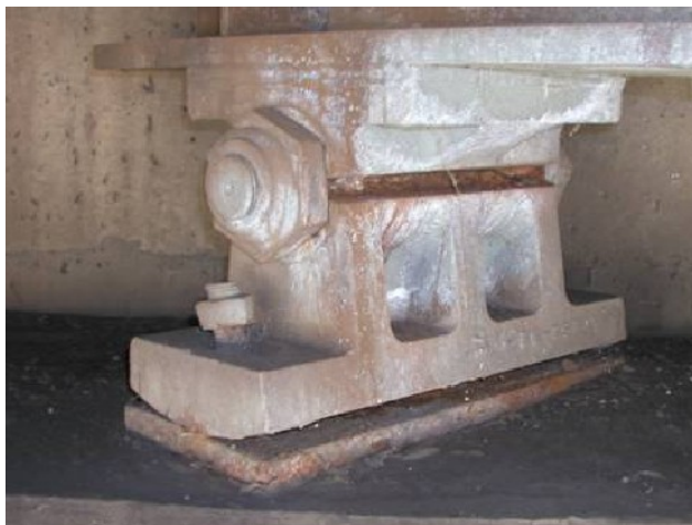
Figure 8 – Uncoated Rocker Assembly Inspection – October 2003
