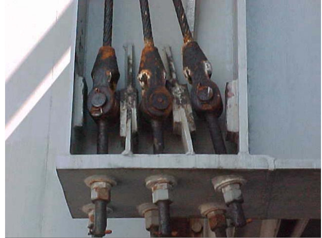
Figure 2 – Typical Corrosion on US Navy Deck Edge Elevator Cables
